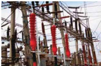
110kV dry style termination installed in Xi'an
